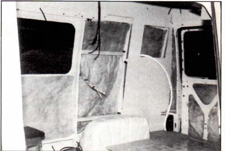
Only Autohomes insulate a panel van this thoroughly (or so they claim) — Talbot Camelot under construction.
