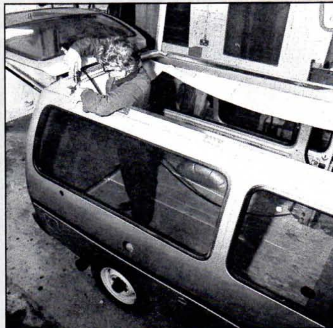
In one corner of the factory is the chassis preparation shop, where roof apertures are cut for van conversions, and where such things as waste tanks and electrical looms are fitted.
